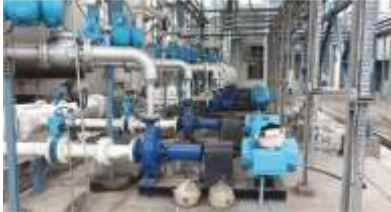
Horizontal end suction pumps
